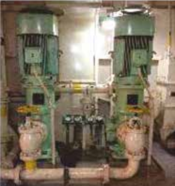
Lubricant oil, 660 gpm / 150 m 3 /h 60 psi / 4 bar Pump installed inside the vessel
