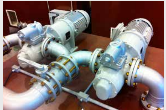
Bearing Lubrication Lubricant Oil 176 gpm / 40 m 3 /h 102 psi / 7 bar
