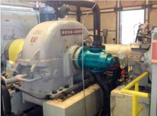
Gear Box Lubrication Lubricant Oil 64.2 gpm / 14.6 m 3 /h 174 psi / 12 bar
