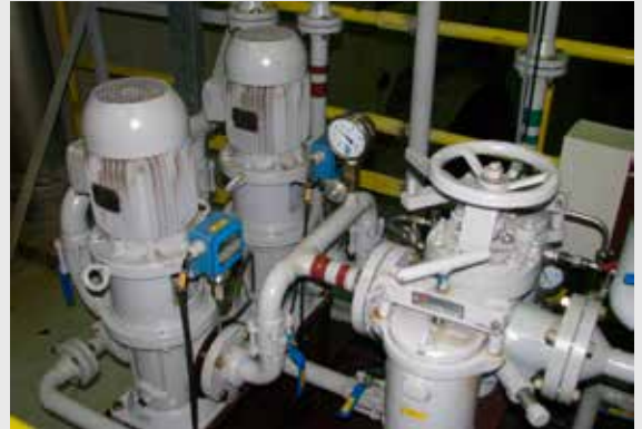
Bearing Lubrication Lubricant Oil 39 gpm / 8.9 m 3 /h 145 psi / 10 bar
