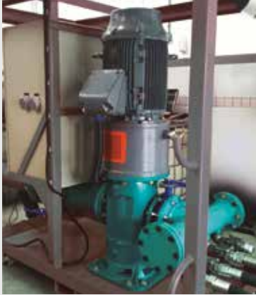
Asphalt Refinery 530 gpm / 120 m 3 /h 150 psi / 10 bar Heating system
